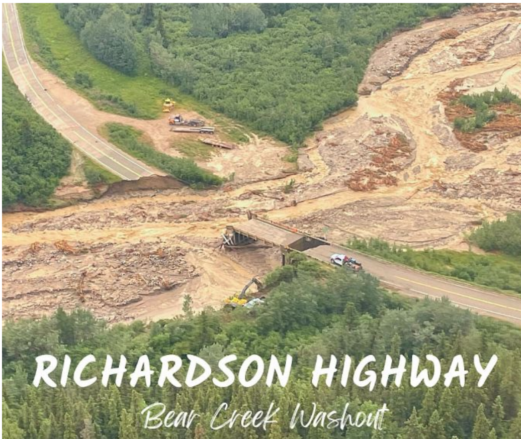
Bear Creek road MP 233 Richardson Highway road washout. Photo by Alyeska Pipeline ( https://dot.alaska.gov/nreg/richardson-washout/ )
